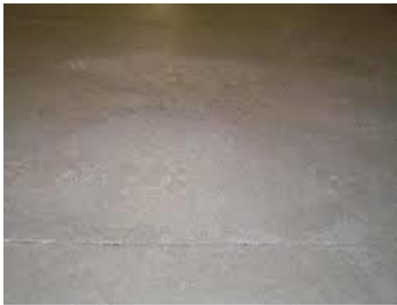
Laitance on concrete
