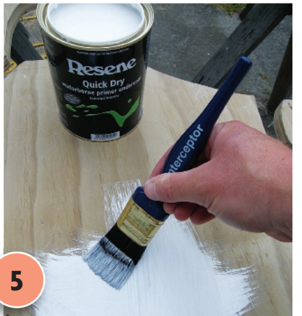
5 Apply a coat of Resene Quick Dry waterborne primer undercoat to the entire gate and allow to dry for two hours.
