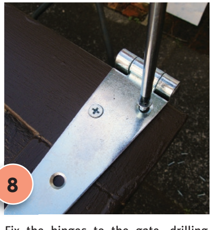
8 Fix the hinges to the gate, drilling pilot holes first, and then position and hang the gate, fixing hinges with remaining screws.
