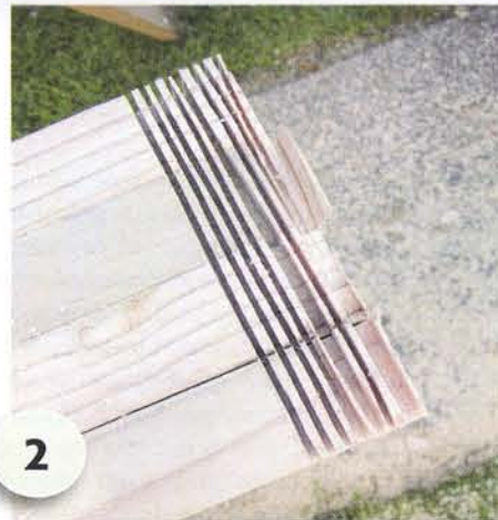
2 Clamp the four legs together. With a framing offcut, mark a line approx 50mm from the top edge. Make a series of cuts, about 25mm deep, across the legs with the circular saw. Knock these through with a hammer; tidy with a chisel. Repeat with the four side and two overhead supports.
