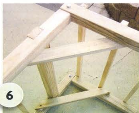
6 Attach side panels to the overhead panel using 50mm x 8mm stainless steel bolts. Use the set square to ensure these are at right angles. Fix with four angled braces cut from the 50mm x 25mm battening. Secure braces with 40mm nails and PVA glue.
