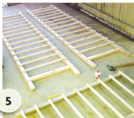
5 Attach the 20mm x 20mm lengths of timber to the side supports and overhead supports, as shown, spacing them about 150mm apart. Use PVA and 40mm nails to fix in position. Leave to dry overnight.
