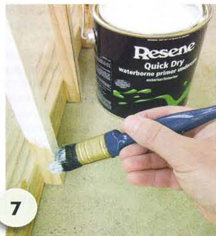
7 Apply one coat of Resene Quick Dry primer undercoat to the entire frame and allow to dry for one hour.
