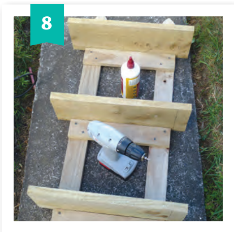
Attach the three 450mm pieces of fence paling to the back frame, as shown, to form the shelves. Fix along the back edge of each shelf with PVA glue and 40mm screws.
