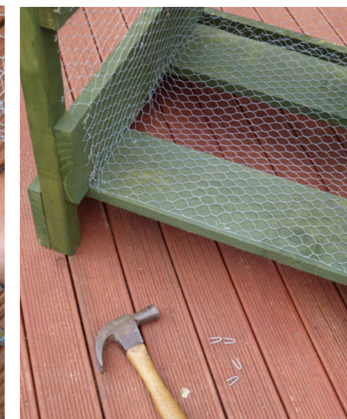
12. Fix the chicken wire into position with galvanised staples. Fix door into position with hinges and fix the catch to keep door closed.
