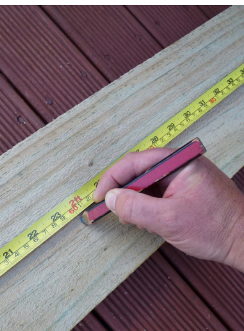
1. Measure and mark each of the fence palings into equal 600mm lengths.
