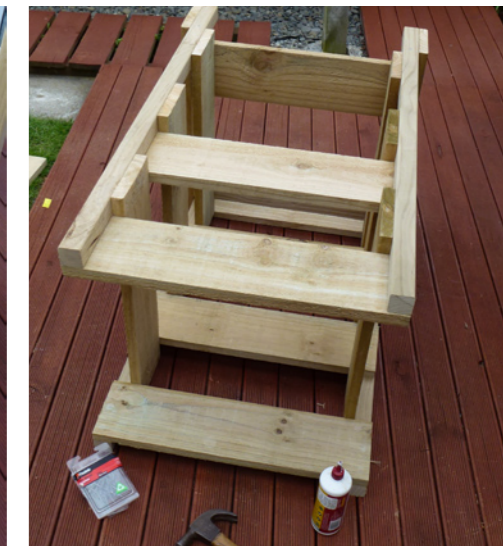
6. In the same way, continue attaching pieces of fence paling to form the front, back and sides of the composter, "staggering" each piece. Leave an opening at the front base of the composter to accommodate the hinged door.
