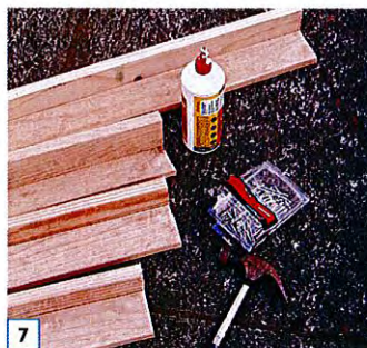
7 Using PVA glue and 50mm nails, fix eight of the 500mm lengths of 70mm x 19mm timber together at right angles to form the corner supports/feet.
