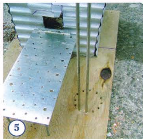
5 HAMMER four galvanised nails into the ply and glue the metal nail plate to the top of each nail to form a platform. Trace around a Resene testpot and, using a hammer and large nail, make 12 holes around the circle. Insert a steel rod into each of these holes with a dab of glue to make the feeding stand.
