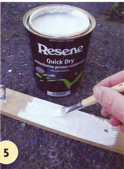
5 Apply a coat of Resene Smooth Surface Sealer to the screw eye and apply one coat of Resene Quick Dry to the wooden bracket.
