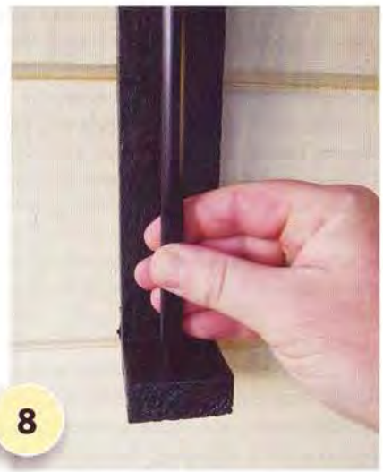
8 Spot prime and paint the bracket screw heads and then hang the lamp on the hook, feeding the pole end through the screw eye and fixing it firmly into the hole in the bottom of the wooden bracket.
