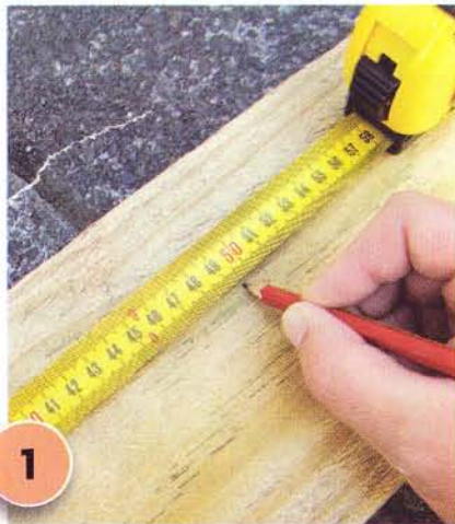
1 Measure the exact width of the wooden panel (ours was actually 495mm) and mark the same measurement on one of the fence palings.
