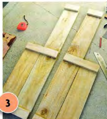
3 Make the sides (as shown) using two 1200mm lengths and two 600mm lengths of rough sawn paling, with four 310mm lengths and the two 155mm lengths of dressed paling. Ensure the ends overlap by approx 25mm; fix with nails and glue.
